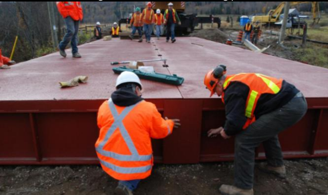
Photo 7: MTO crew and construction forces attach soil retention plates following the connection of section 1 to section 2 of the bridge.
