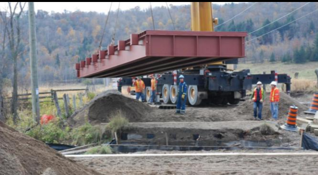
Photo 3: Section 1 of new 18.3m span Lessard Modular Bridge is hoisted by 90 ton crane into position. New concrete bearing visible in foreground.
