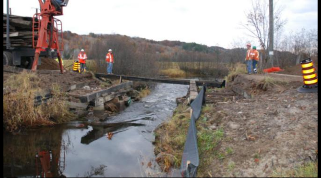
Photo 2: Upstream face of Bass Lake Creek Crossing. New concrete bearing substructure is visible upper right. Old stringers provide temporary for access for construction crew.
