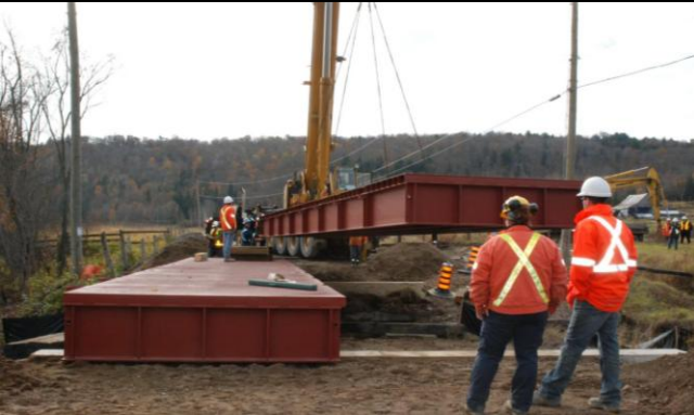
Photo 5: Section 1 (upstream face) in final position, Section 2 of new 18.3m span Lessard Modular bridge is lowered into matching position.
