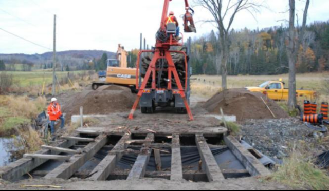
Photo 1: Logging Truck, together with Case track excavator remove decking of existing bridge, exposing decayed 300mm timber stringers.
