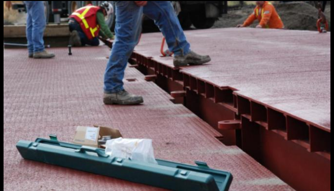
Photo 6: Construction forces guide the tie down plates of Section 2 to the receiving plates on Section 1 and connect using structural bolts.
