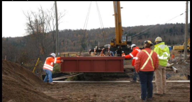
Photo 4: Section 1 (upstream face) is lowered carefully into position. Concrete bearing swept clear of debris prior to final section location.
